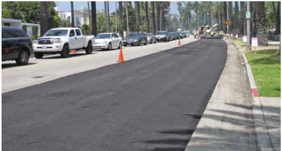
Maintaining uninterrupted traffic was critical to the project. The prime and recycling contractors had to maintain two lanes of traffic at all times, and residents were granted 100% access in and out of the work site.
